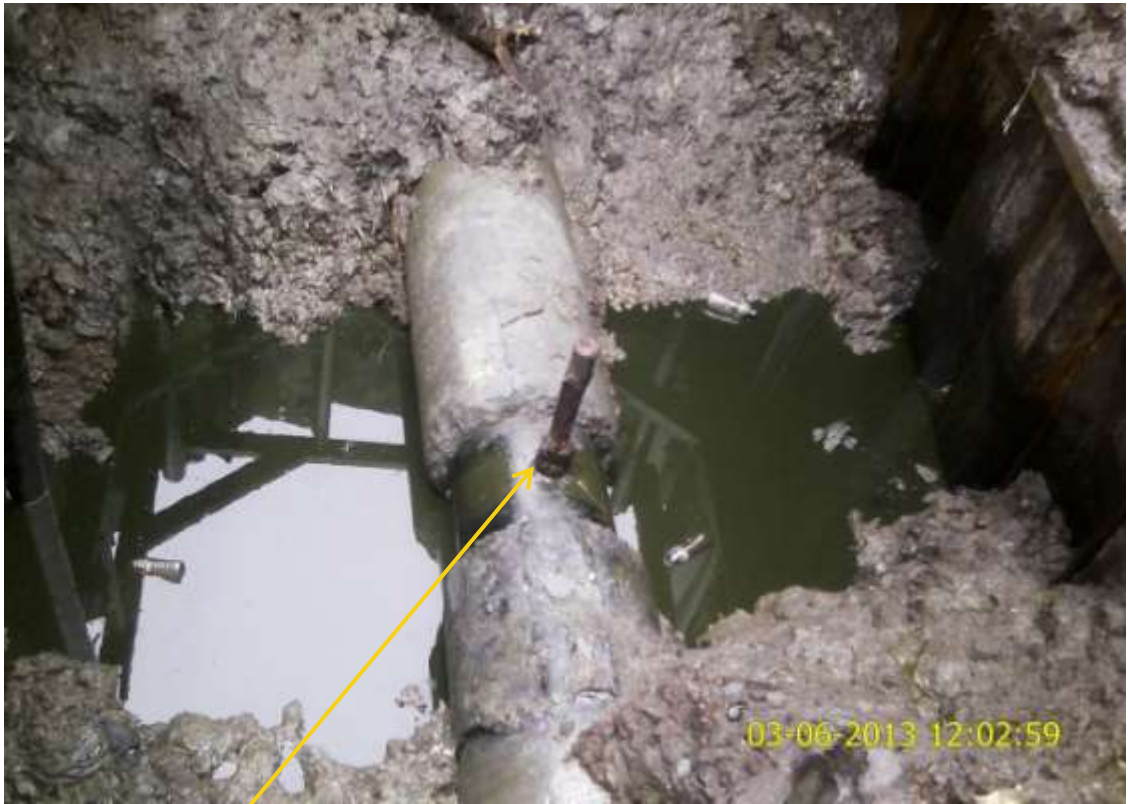
Close up: Illegal fitting on 24" Nem,be creek pipeline at Adamakiri. Picture was taken during Joint Investigation of 3 rd June 2013.
