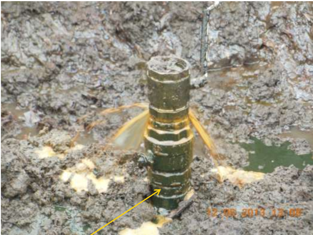
Close up: Illegal fitting on 28" Bomu-Bonny Trans Niger pipeline at Bodo West. Picture was taken during Joint Investigation of 12 th June 2013.
