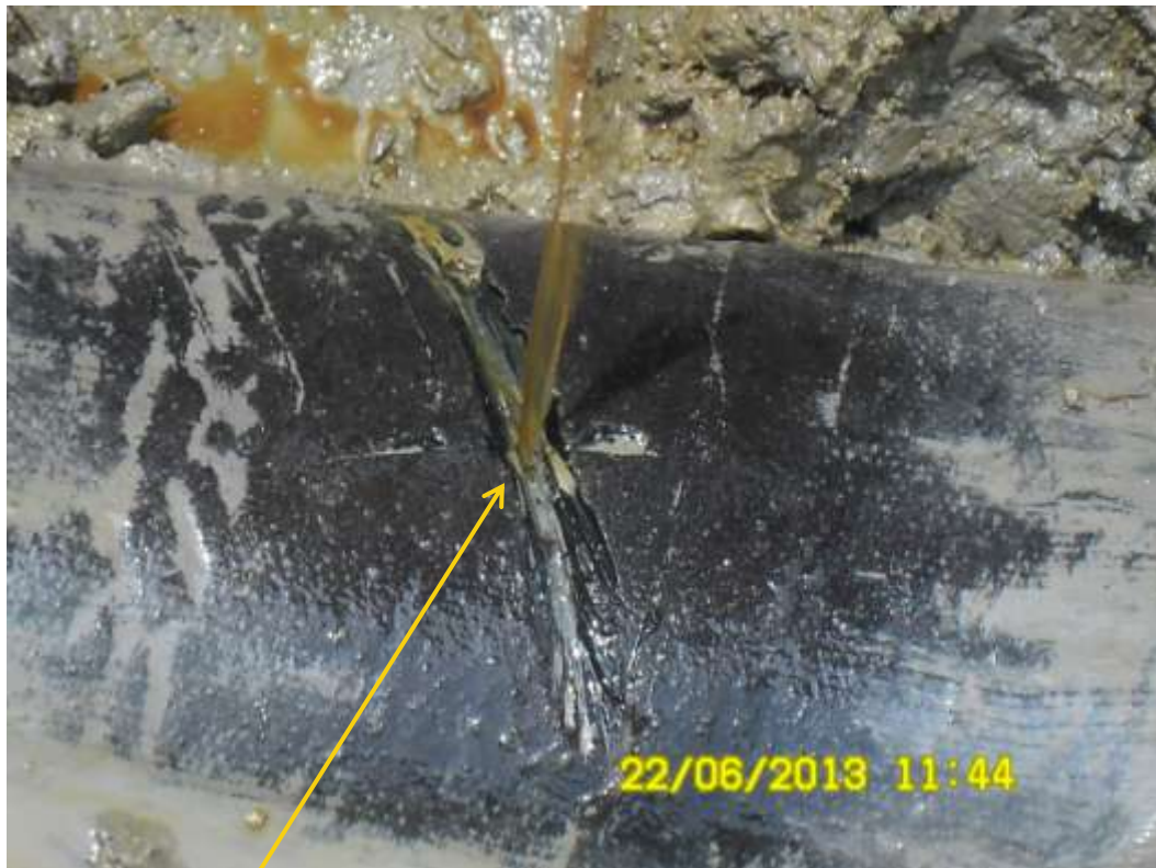
Close up: Hacksaw cut on 10" Diebu Creek – Nun River pipeline at Onyoma/Eniwari. Picture was taken during Joint Investigation of 22 nd June 2013.
