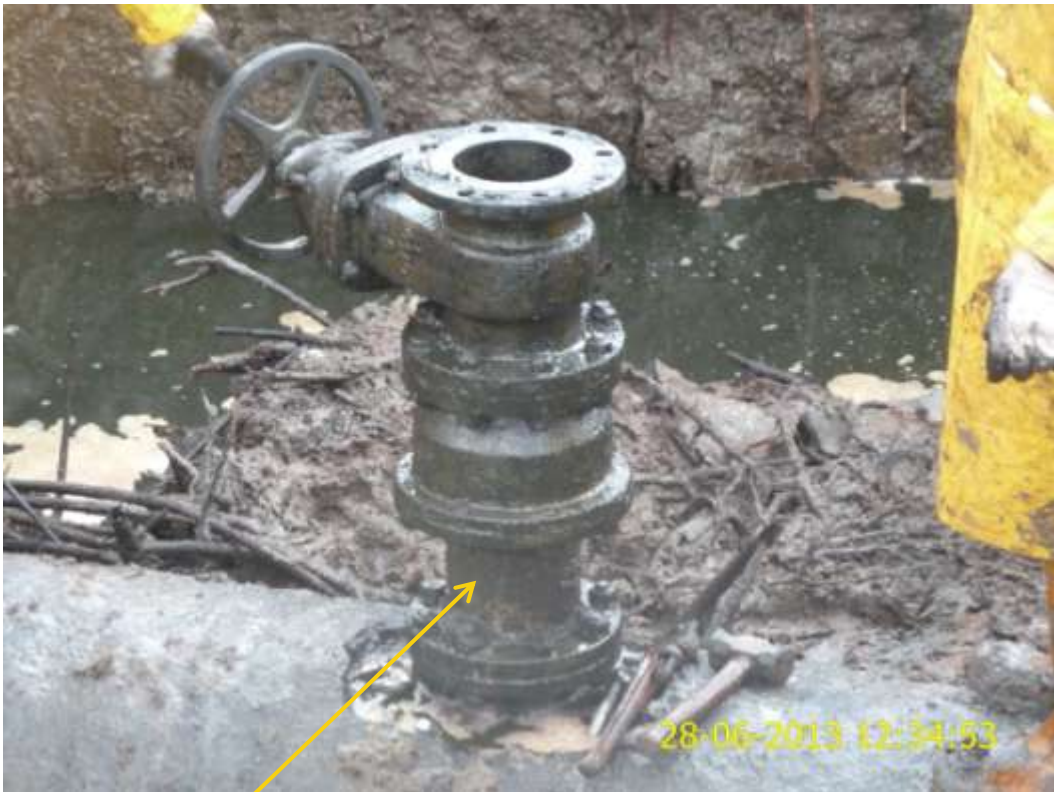
Close up : Illegal fitting on 28" Bomu-Bonny Trans Niger pipeline at Bodo West. Picture was taken during Joint Investigation of 28 th June 2013.
