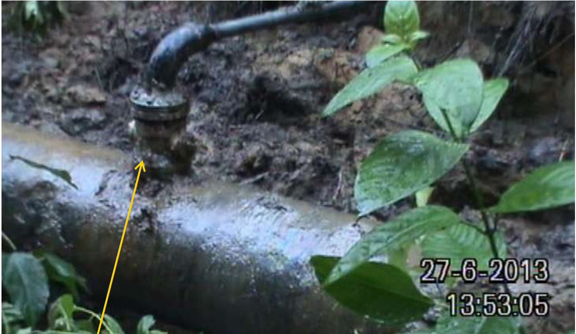
Close up: Illegal fitting on 20" Otumara-Escravos trunkline at Adjudaibo. Picture was taken during Joint Investigation of 27 th June 2013.
