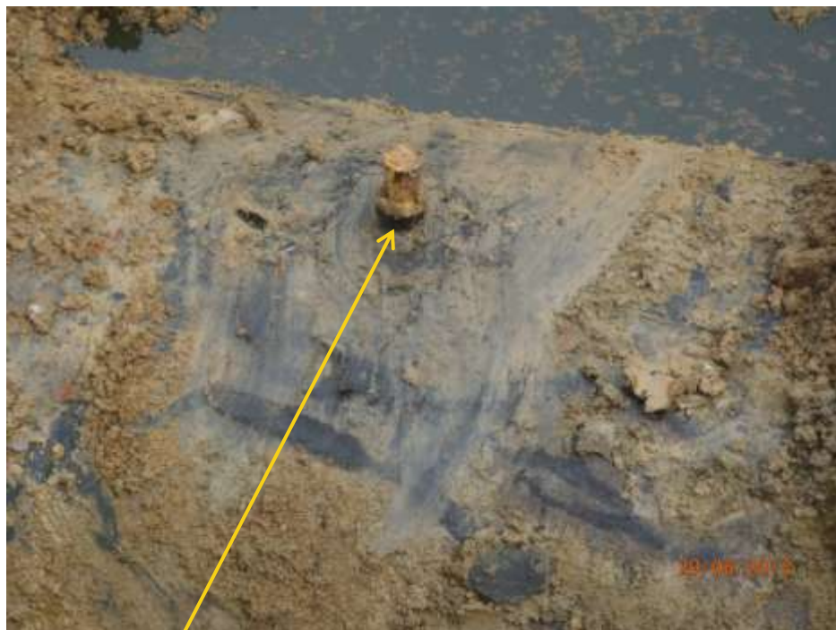
Close up: Illegal fitting on 36" Rumuekpe-Nkpoku pipeline at Omujiewhor-Ibaa. Picture was taken during Joint Investigation of 29 th June 2013.
