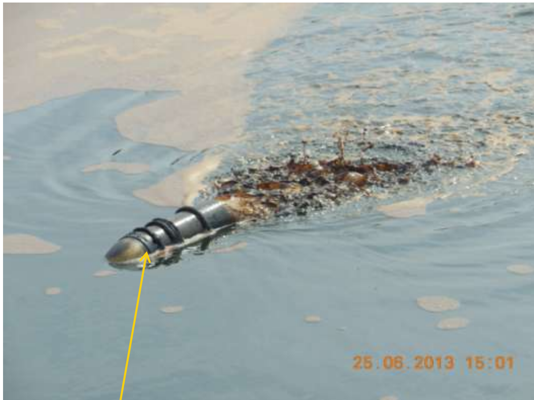
Close up: Illegal fitting on 28" Bomu-Bonny Trans Niger pipeline at BodoWest. Picture was taken during Joint Investigation of 25 th June 2013.
