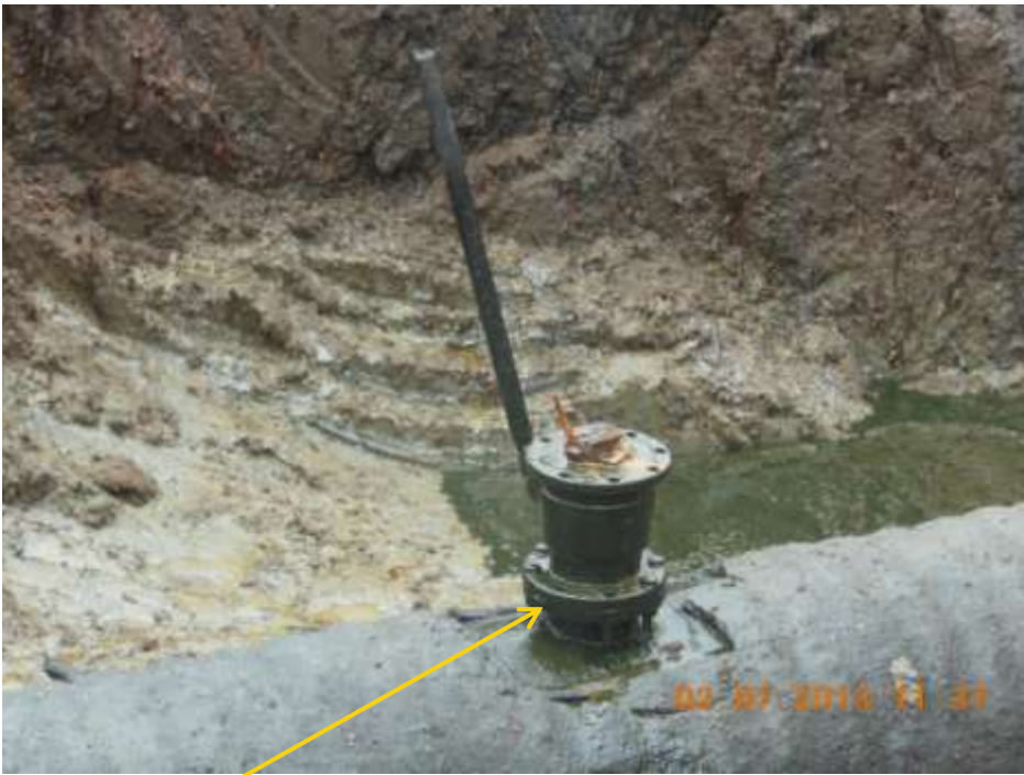
Close up: 28" Bomu-Bonny Trans Niger pipeline at Bodo West. Picture was taken during Joint Investigation of 2 nd July 2013.
