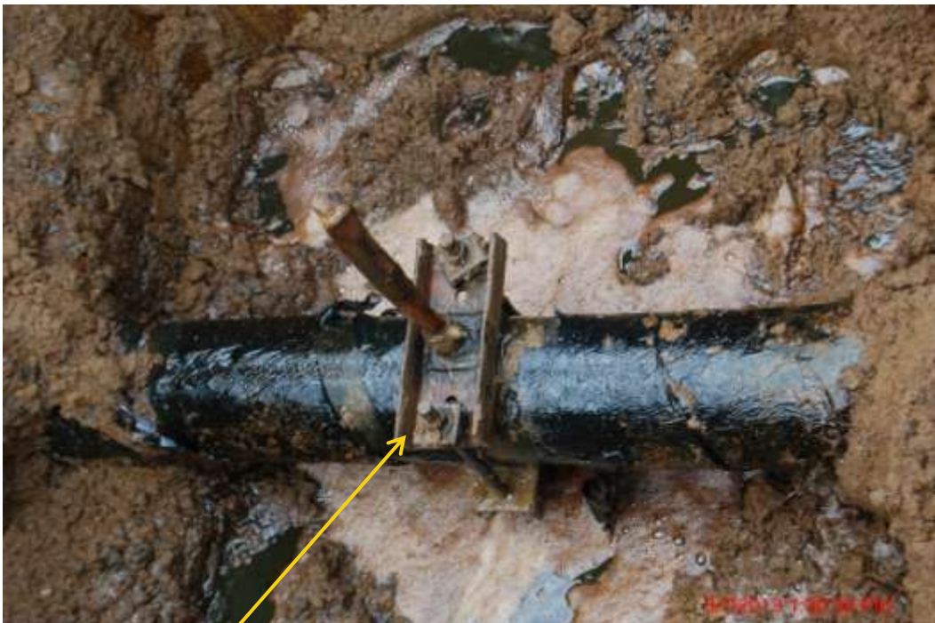
Close up: Illegal fitting on 6" Obigbo North – Ogale pipeline at Ogale. Picture was taken during Joint Investigation of 3 rd July 2013.
