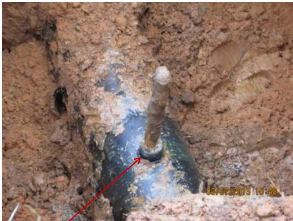
Close up: Illegal fitting on 12" Oguta-Egbema pipeline at Obiakpu. Picture was taken during Joint Investigation of 3 rd July 2013.
