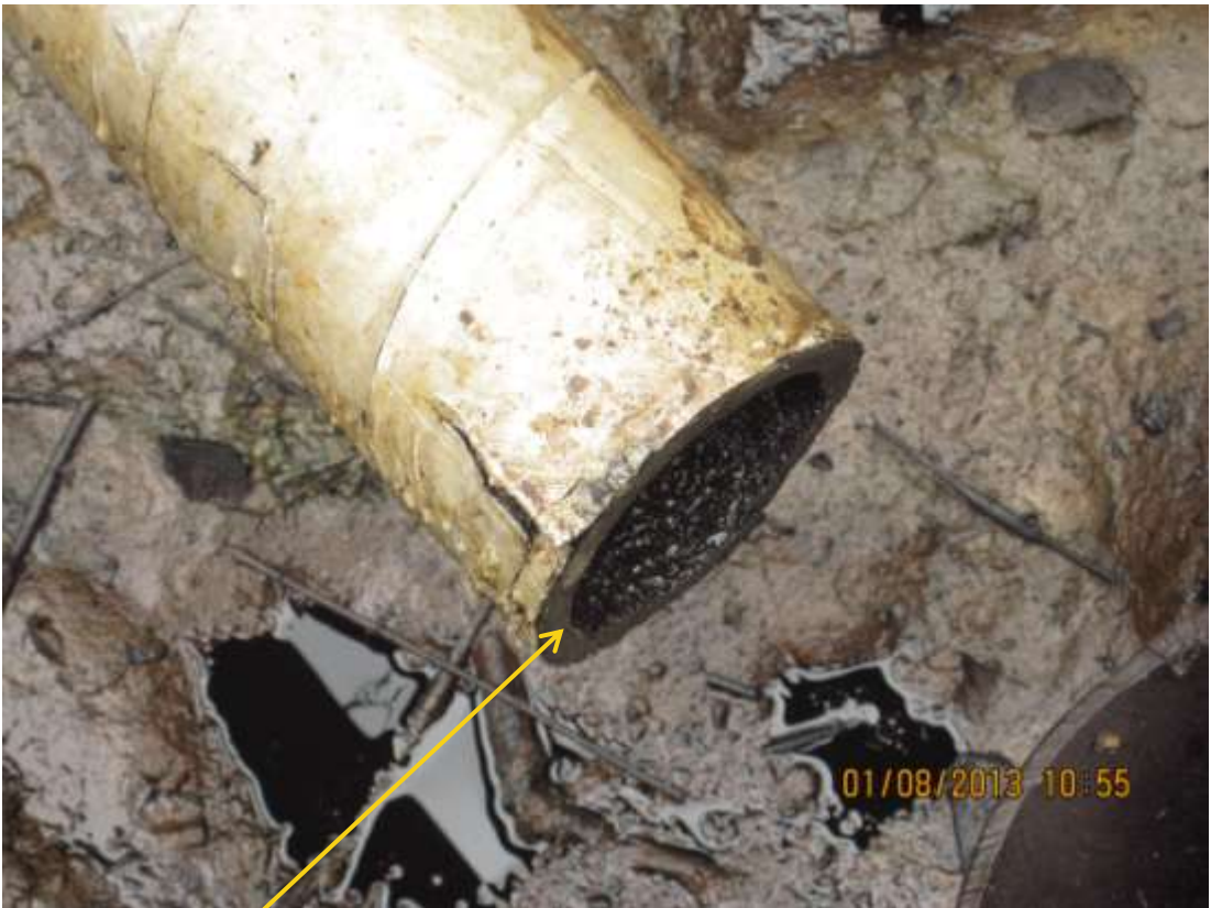
Close up: Cut section on 3" Imo River Well5L flowline at Igiriukwu. Picture was taken during Joint Investigation of 1 st August 2013.
