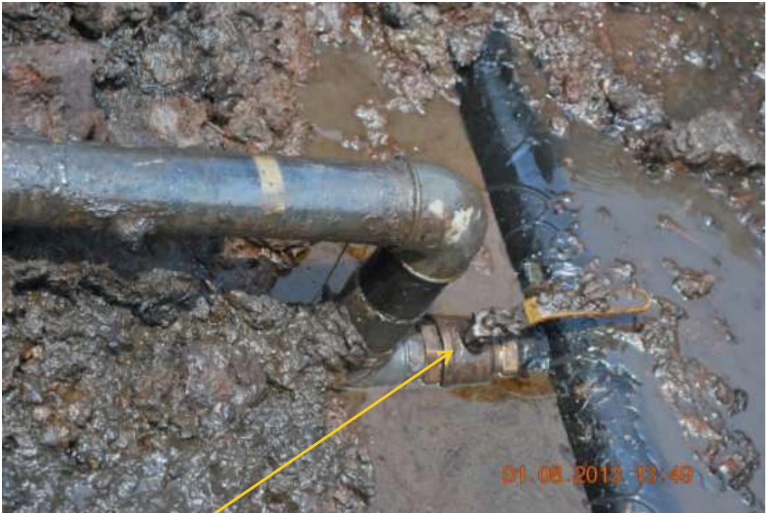
Close up: Illegal fitting on 6" Cawthorne Channel3 Well4S at Krakrama. Picture was taken during Joint Investigation of 1 st August 2013.
