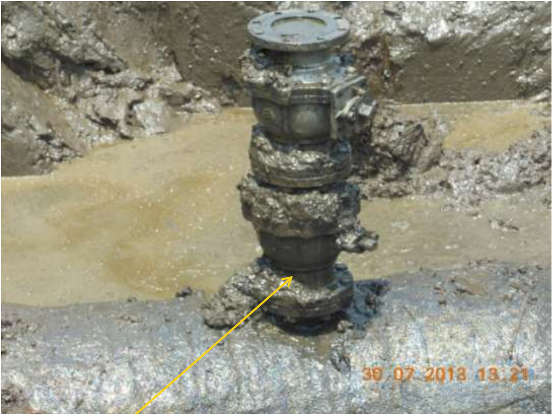
Close up : Illegal fitting on 28" Bomu-Bonny TransNiger pipeline at Freetown. Picture was taken during Joint Investigation of 30 th July 2013.
