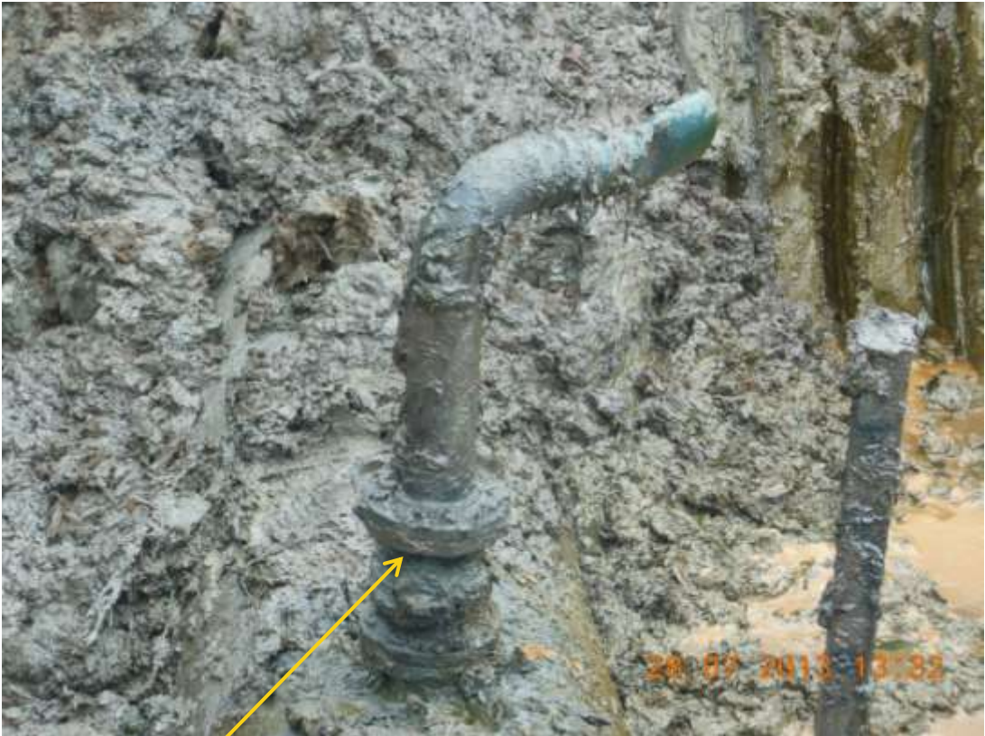
Close up: Illegal fitting on 28" Bomu-Bonny TransNiger pipeline at Freetown. Picture was taken during Joint Investigation of 28 th July 2013.
