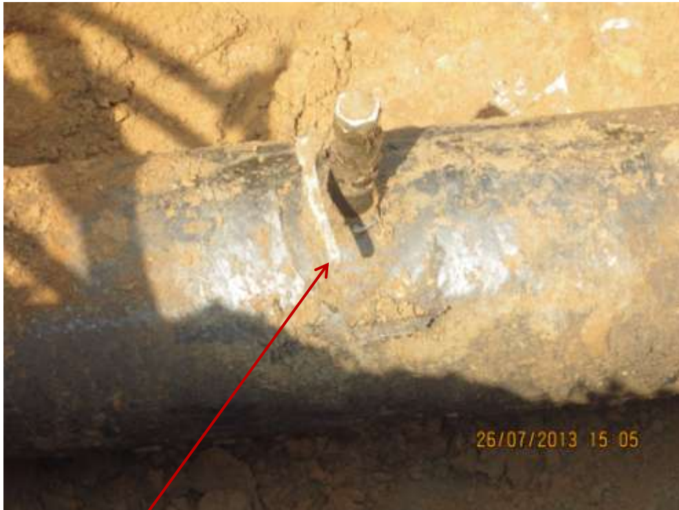
Close up: Illegal fitting on 12" Imo River2 – Ogale pipeline at Etituzo/Owaza. Picture was taken during Joint Investigation of 26 th July 2013.
