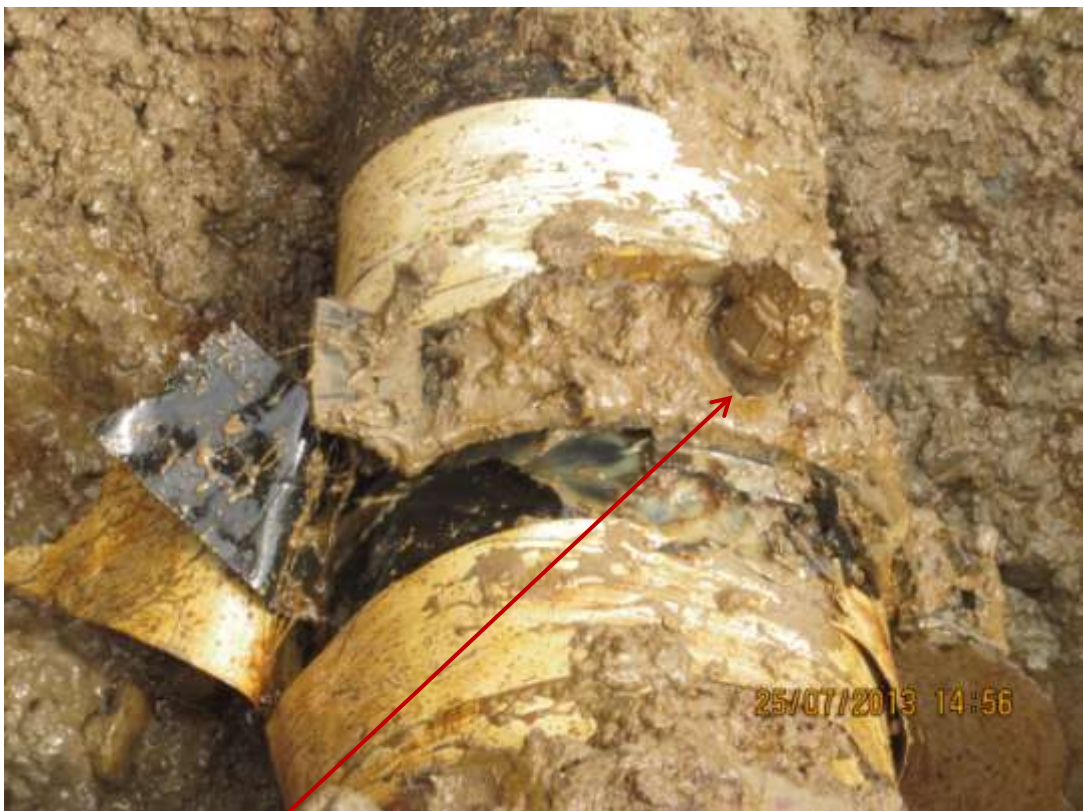
Close up: Illegal fitting on 12" Imo River2 – Ogale pipeline at Umuedeokwara /Odagwa. Picture was taken during Joint Investigation of 25 th July 2013.
