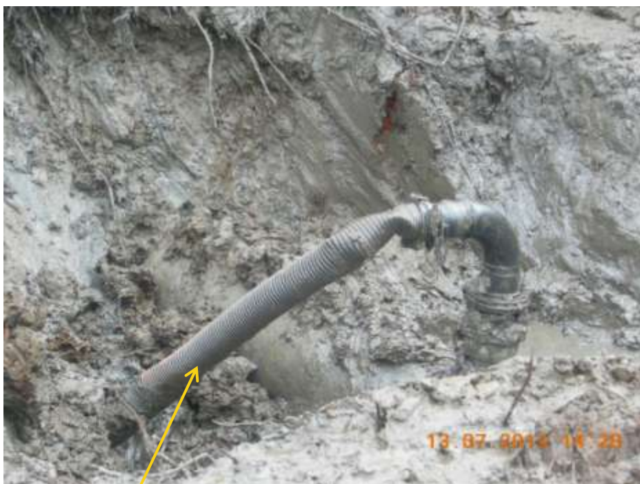
Close up: Illegal fitting on 24" Bomu-Bonny Trans Niger pipeline at Owokiri-Bodo. Picture was taken during Joint Investigation of 13 th July 2013.
