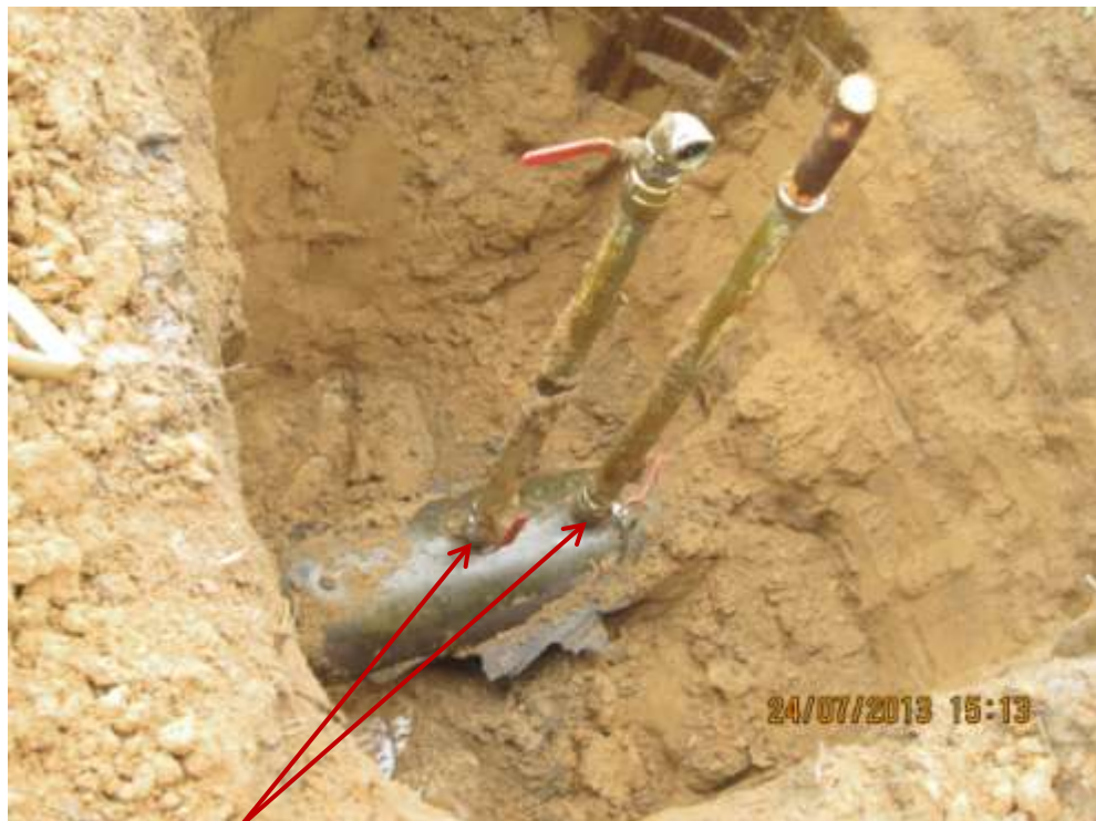
Close up: Illegal fittings on 12" Imo River2 – Ogale pipeline at Umuololo/Owaza. Picture was taken during Joint Investigation of 24 th July 2013.
