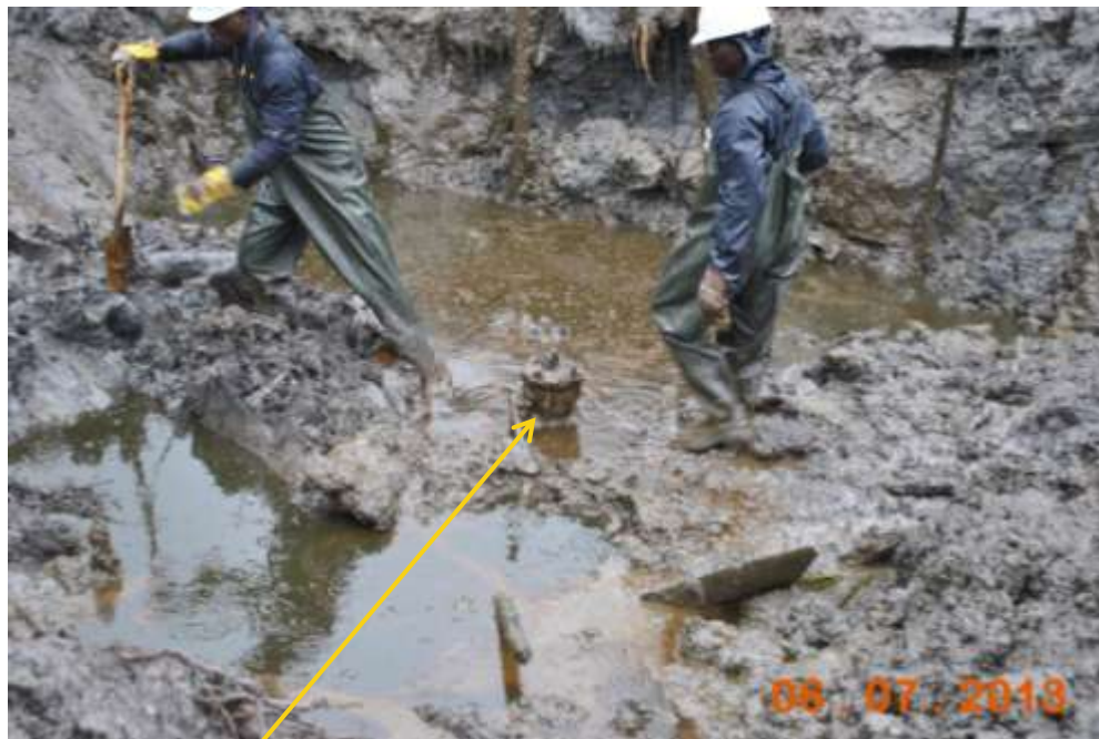
Close up: Illegal fitting on 20" Otumara-Escravos pipeline at Otumara. Picture was taken during Joint Investigation of 6 th July 2013.
