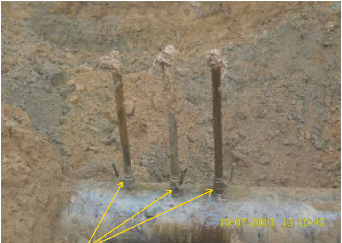
Close up: Illegal fittings on 24" Nkpoku-Bomu pipeline at Rumuoegwu-Eneka. Picture was taken during Joint Investigation of 10 th July 2013.
