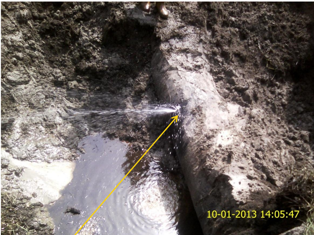
Close up: Spill due to hacksaw cut on 24" Bomu-Bonny pipeline at Mogho. Picture was taken during Joint Investigation of 10 th January 2013.
