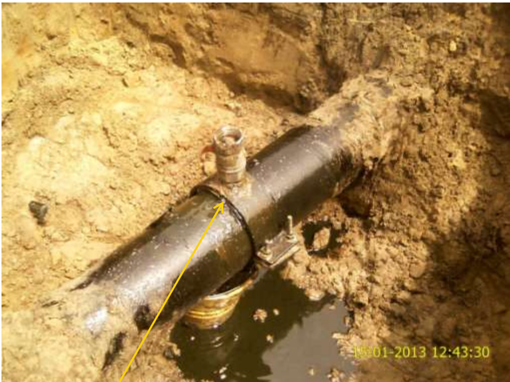
Close up: Illegal fitting on 8" Isimiri-Imogate pipeline at Uzuaku. Picture was taken during Joint Investigation of 15 th January 2013.
