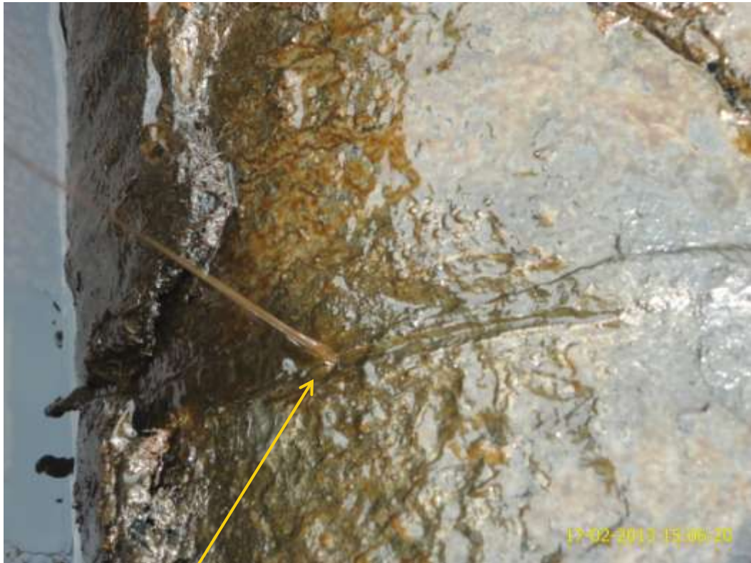
Close up: Ground off welding joint on 10" Ekulama-Sanbarth pipeline at New Town. Picture was taken during Joint Investigation of 17 th February 2013.
