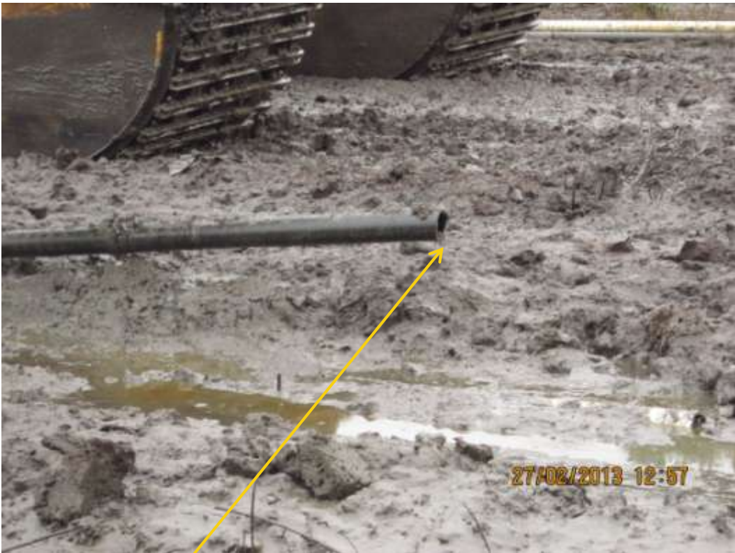
Close up: Missing flowline section on Nembe 2 Well17S flowline at Nembe. Picture was taken during Joint Investigation of 27 th February 2013.
