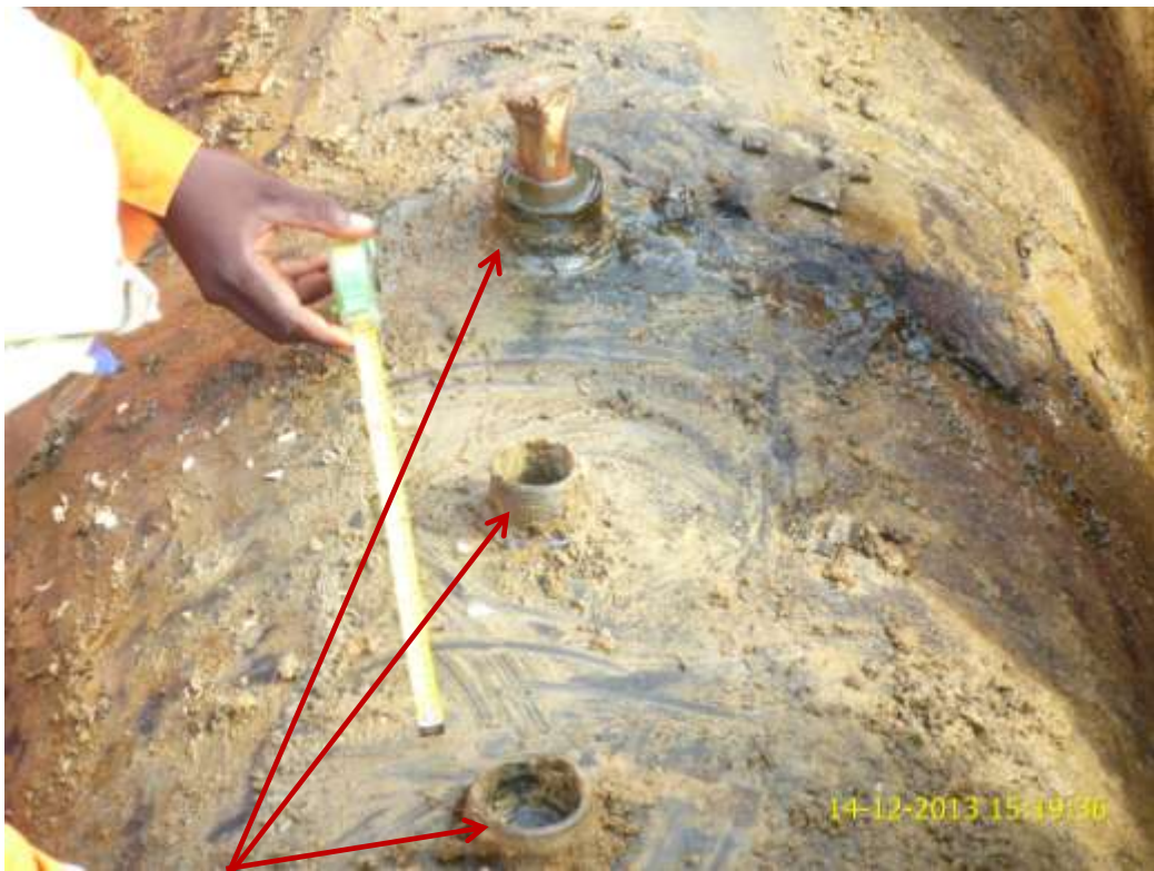
Close-up: Illegal fittings on 36" Nkpoku-Bomu Pipeline at Agbonchia. Picture was taken during Joint Investigation of 14 th December 2013.
