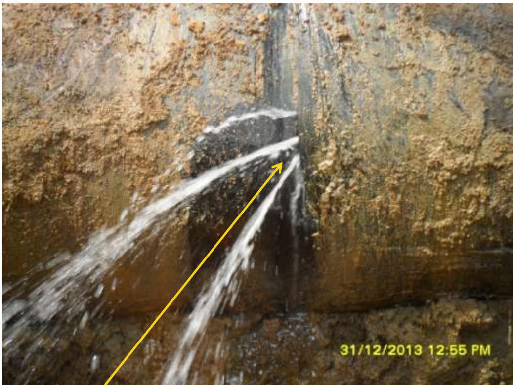
Close-up: Hacksaw cut on 24" Nkpoku – Bomu Pipeline at Kpите. Picture was taken during Joint Investigation of 31st December 2013.
