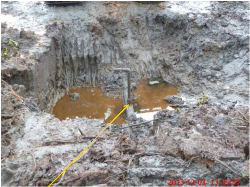
Close-up: Illegal fitting on 6" Awoba flowstation Manifold Pipeline at Awoba. Picture was taken during Joint Investigation of 3 rd December 2013.
