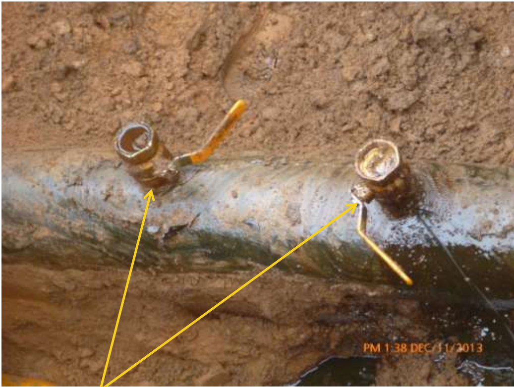
Close-up: Illegal fittings on 8" Obigbo North – Ogale Pipeline at Umosoya. Picture was taken during Joint Investigation of 11 th December 2013.
