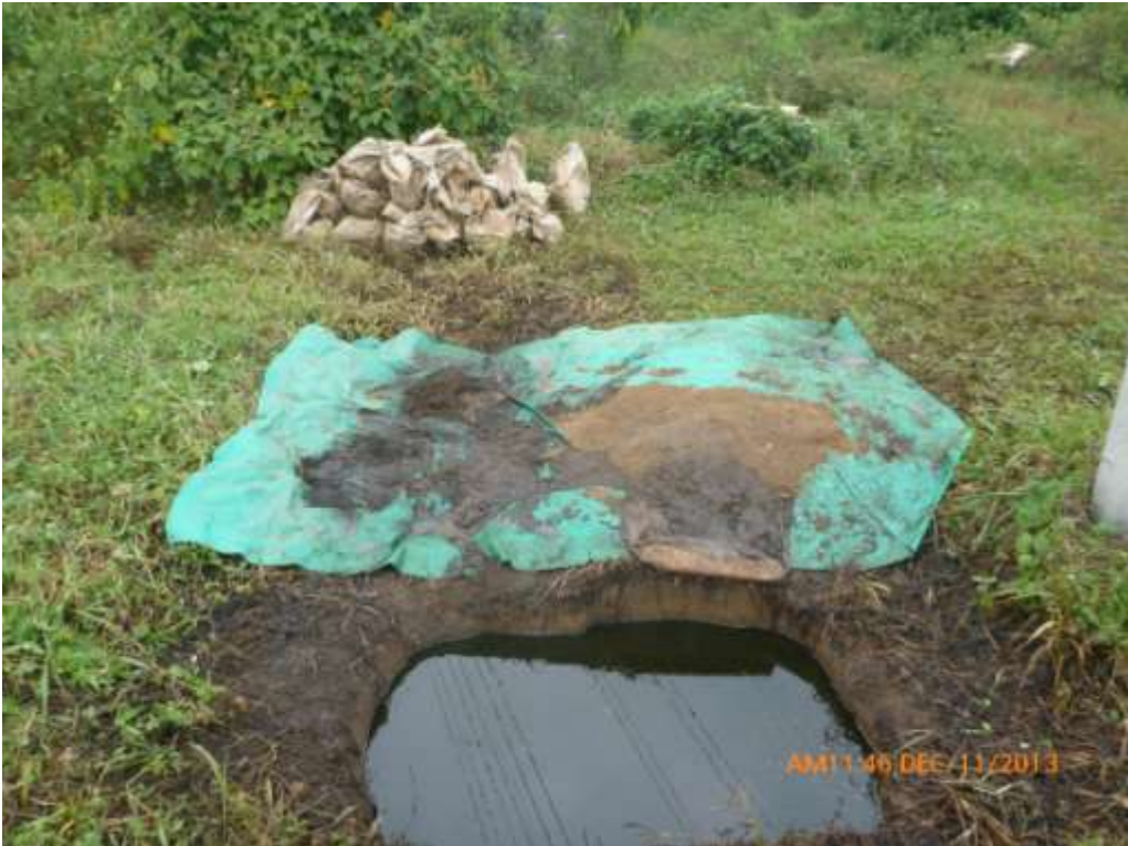
Overview: Part of spill impact on 8" Obigbo North – Ogale Pipeline right of way at Umosoya. Picture shows sandbags and tarpaulin left behind by unknown persons. Picture was taken during Joint Investigation of 11th December 2013.
