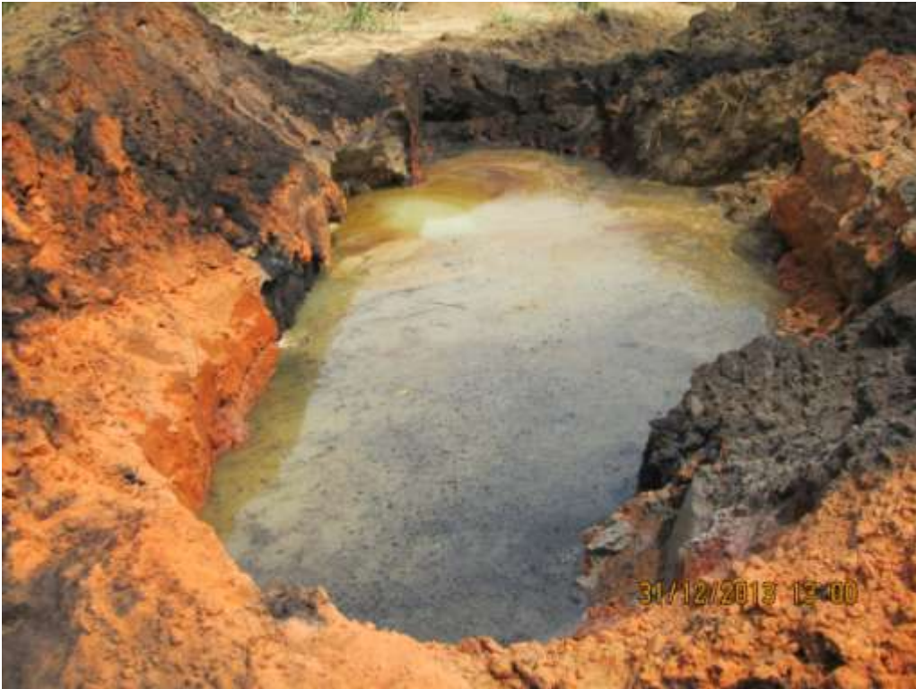
Overview: Part of spill impact on 28" Nkpoku – Bomu Pipeline right of way at B-Dere. Picture was taken during Joint Investigation of 31 st December 2013.
