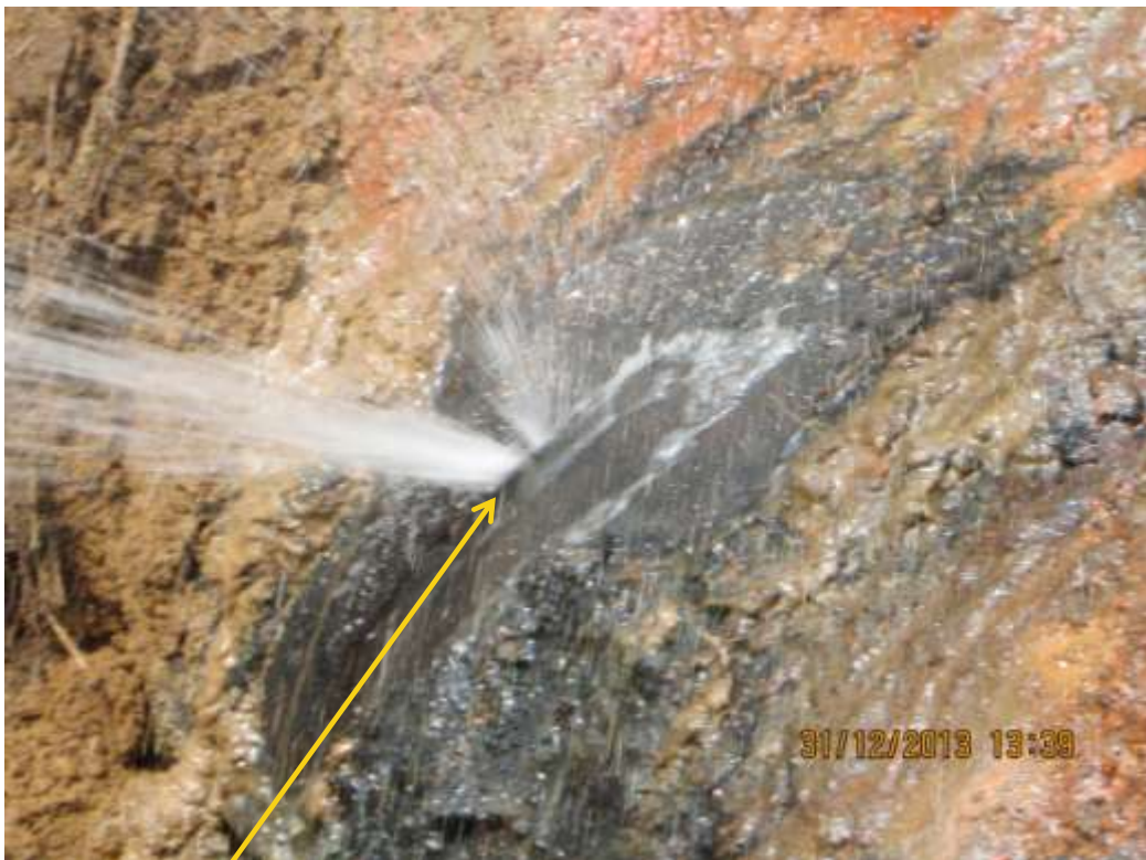
Close-up: Hacksaw cut on 28" Nkpoku – Bomu Pipeline at B-Dere. Picture was taken during Joint Investigation of 31 st December 2013.
