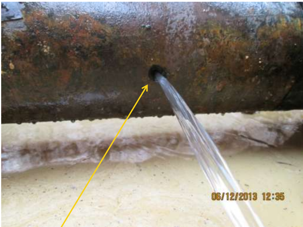
Close-up: Spill due to corrosion on 6" Obigbo North – Ebubu Pipeline at Obolo. Picture was taken during Joint Investigation of 6 th December 2013.
