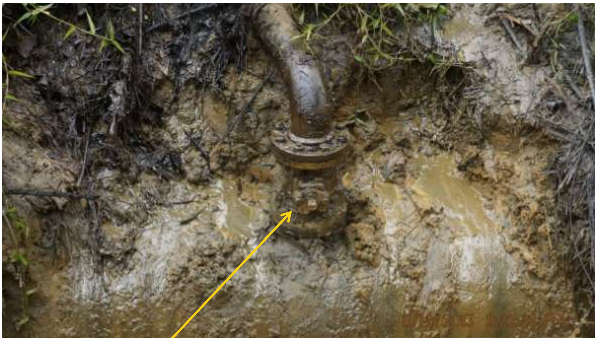
Close-up: Illegal fitting on 20" Otumara - Escravos Pipeline at Ogidigben. Picture was taken during Joint Investigation of 11th December 2013.
