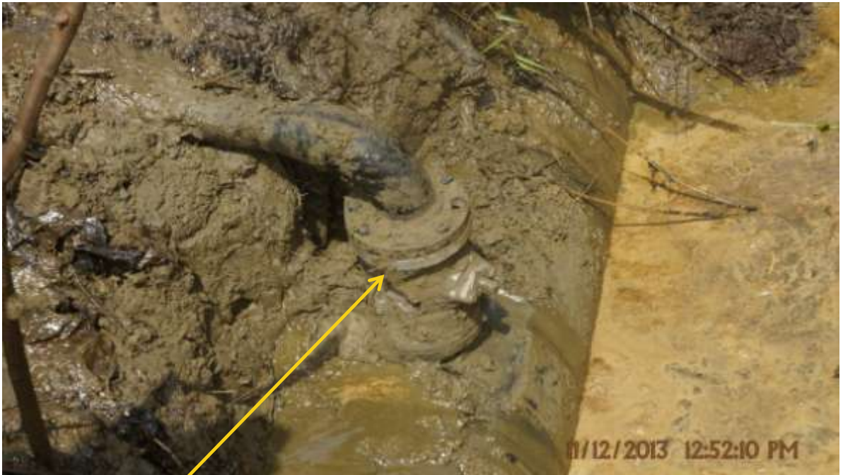
Close-up : Illegal fitting on 20" Otumara - Escravos Pipeline at Ogidigben. Picture was taken during Joint Investigation of 11 th December 2013.
