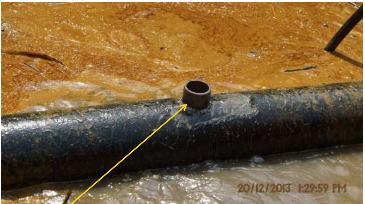
Close-up: Illegal fitting on Seibou Bulkline3 at Azargbene. Picture was taken during Joint Investigation of 20th December 2013.
