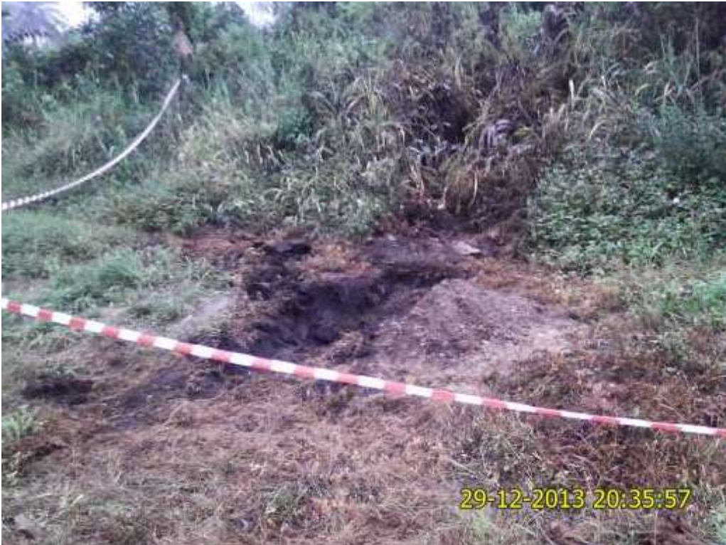
Overview: Part of spill impact on 12" Oguta – Egbema Pipeline right of way at Obiakpu. Picture was taken during Joint Investigation of 29th December 2013.
