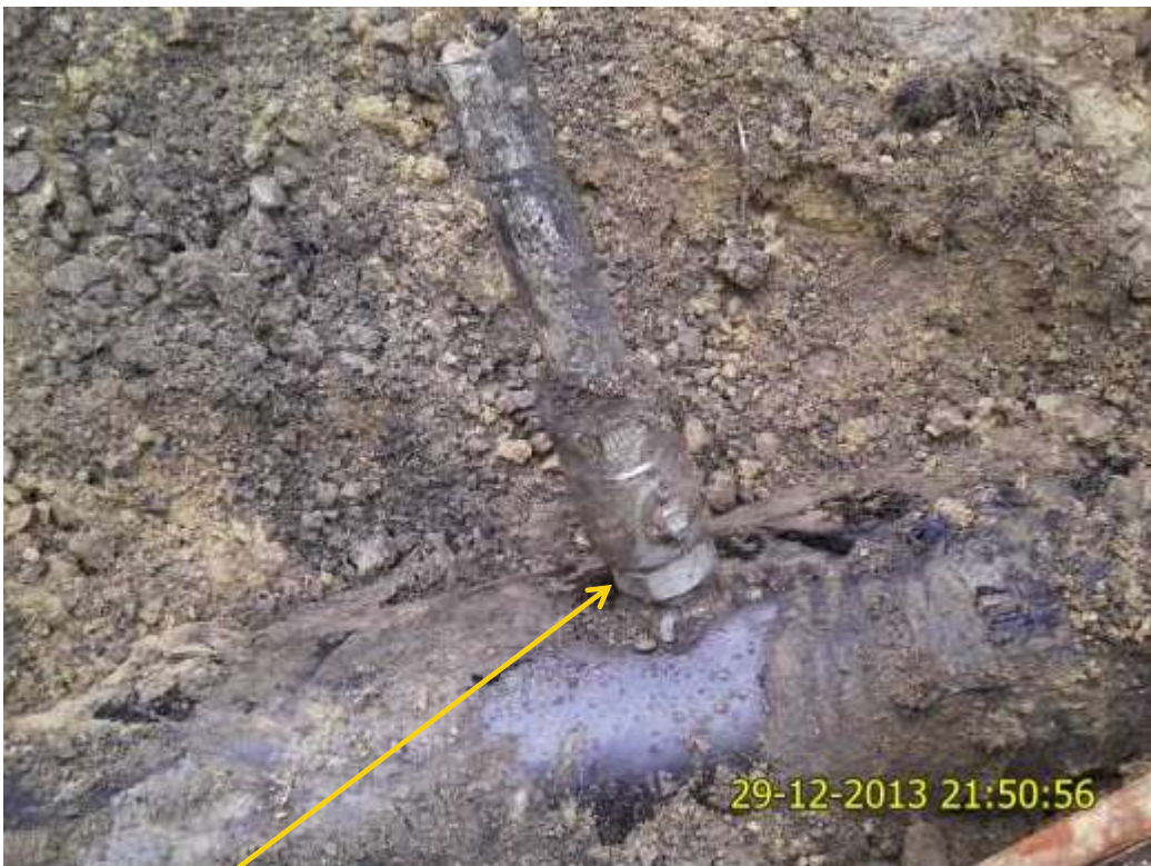
Close-up: Illegal fitting on 12" Oguta – Egbema Pipeline at Obiakpu. Picture was taken during Joint Investigation of 29th December 2013.
