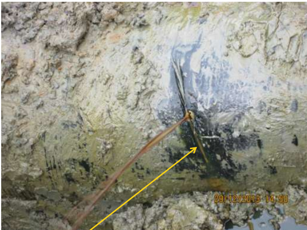
Close-up: Hacksaw cut on 16" Nunriver – Kolocreek Pipeline at Oporoma. Picture was taken during Joint Investigation of 29 th December 2013.
