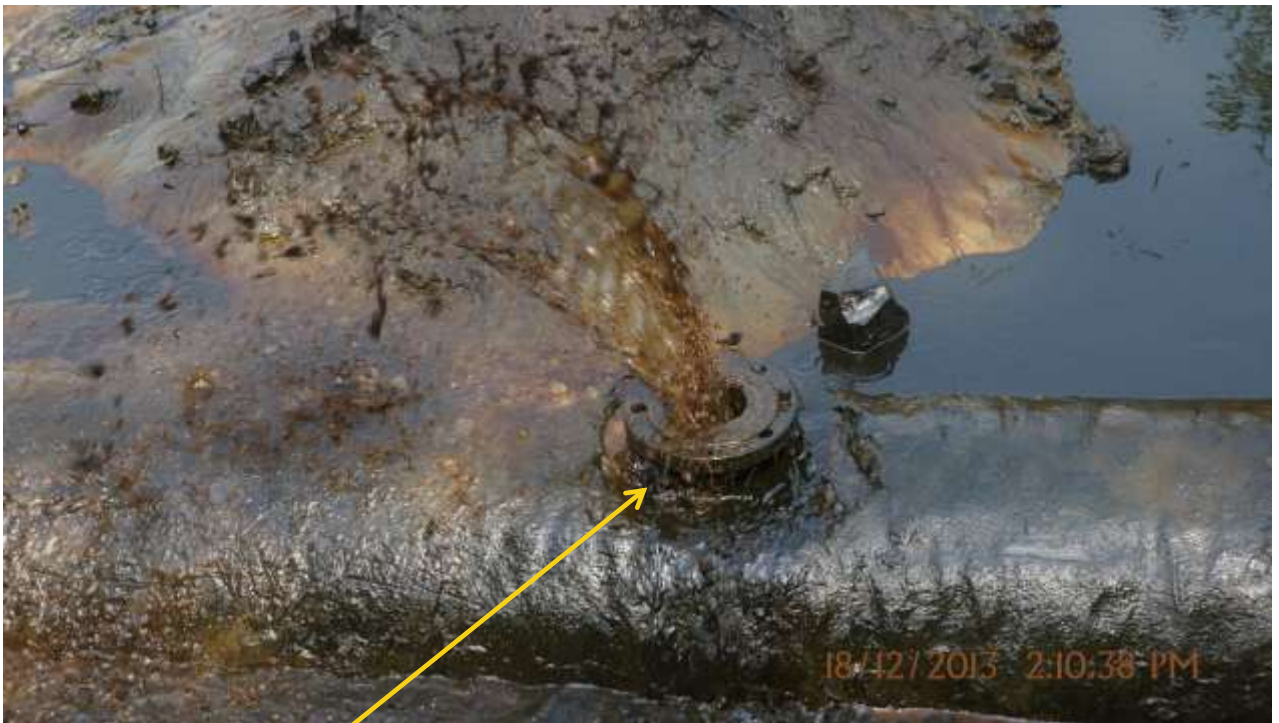
Close-up: Illegal fitting on 20" Otumara – Escravos Pipeline at Ugboegungun. Picture was taken during Joint Investigation of 18th December 2013.
