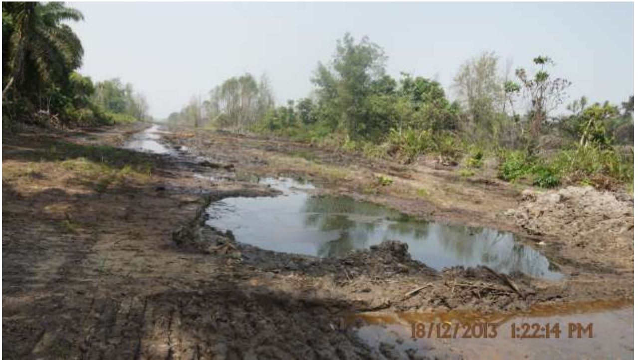
Overview: Part of spill impact on 20" Otumara – Escravos Pipeline right of way at Ugboegungun. Picture was taken during Joint Investigation of 18th December 2013.
