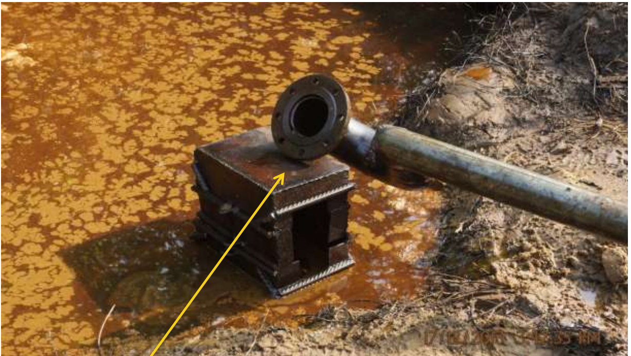
Close-up: Illegal fitting on 20" Otumara – Escravos Pipeline at Adjudaibo. Picture was taken during Joint Investigation of 17 th December 2013.
