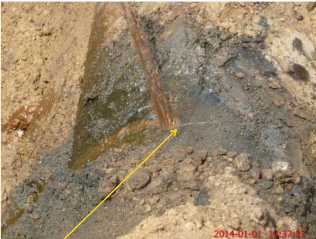
Close-up: Hacksaw cut on 24" Bomu-Bonny Trans Niger Pipeline at Mogho. Picture was taken during Joint Investigation of 1st January 2014.
