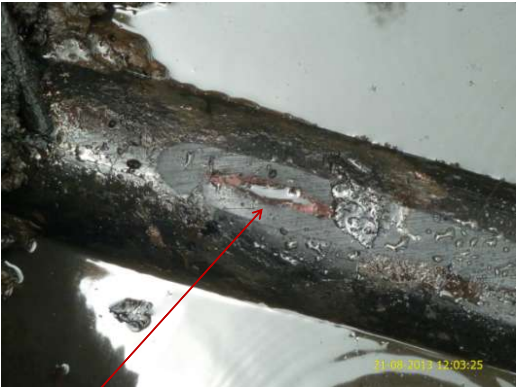
Close up: Damage from heavy equipment on 4" Cawthorne Channel Well51T flowline at Mbiama. Picture was taken during Joint Investigation of 21 st August 2013.
