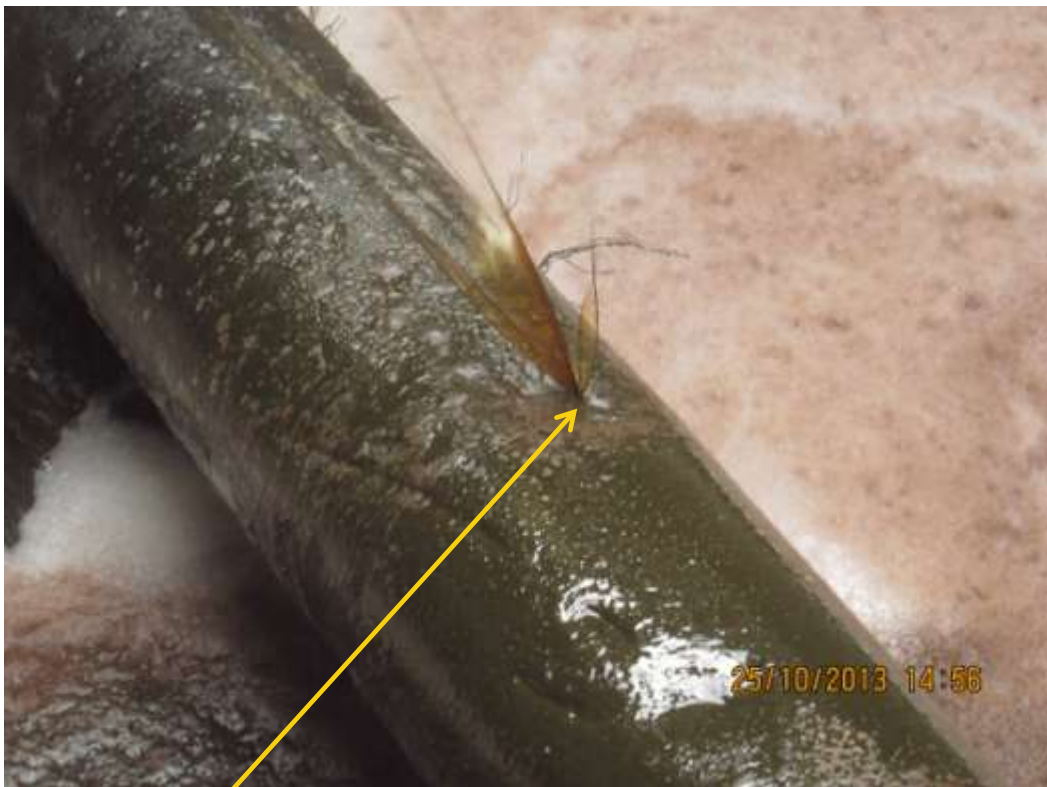
Close-up: Spill due to corrosion on 10" Ekulama1 – Sanbarth Pipeline at Ekulama. Picture was taken during Joint Investigation of 25th October 2013.
