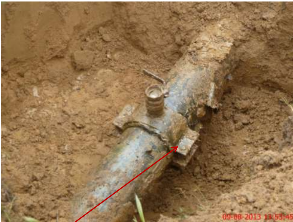
Close up: Illegal fitting on 8" Isimiri-Imo River pipeline at Obiakpu. Picture was taken during Joint Investigation of 9 th August 2013.
