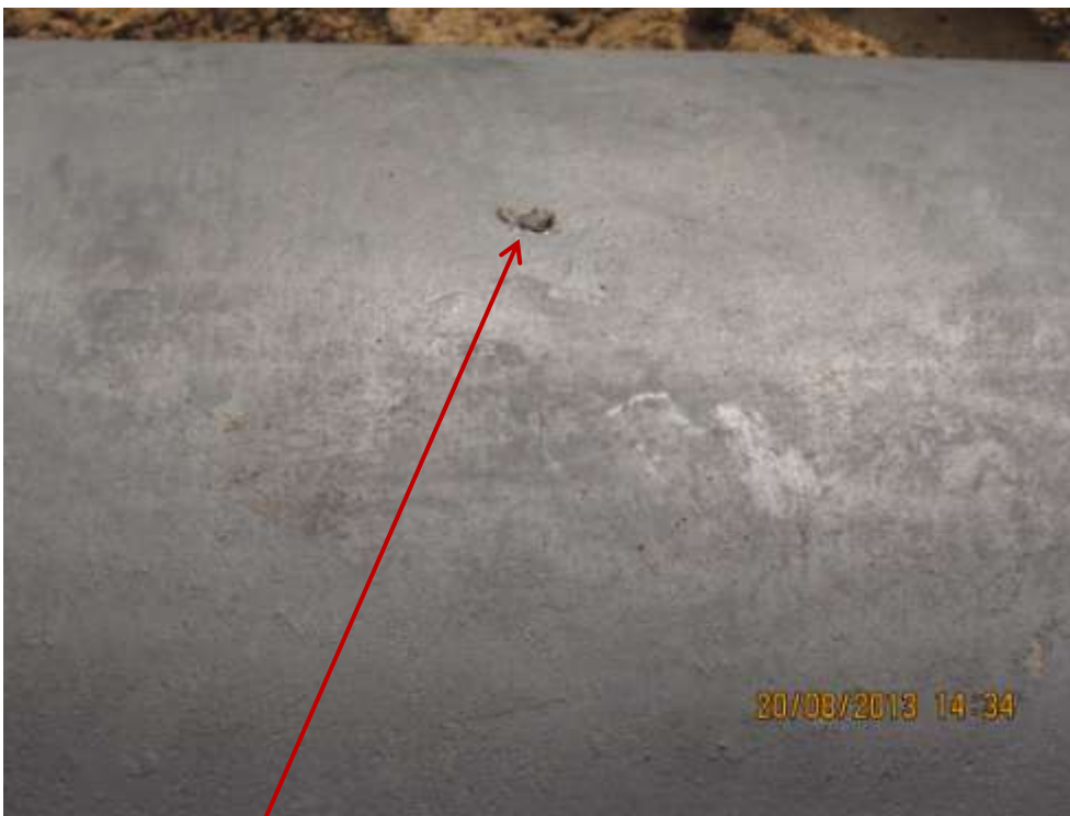
Close up: Drilled hole on 24" Nkpoku-Bomu Trans Niger pipeline at Bera. Picture was taken during Joint Investigation of 20 th August 2013.
