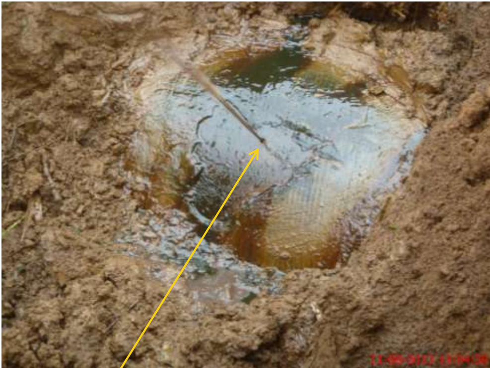
Close up: Drilled hole on 24" Npoku-Bomu Trans Niger pipeline at Biara. Picture was taken during Joint Investigation of 11 th August 2013.
