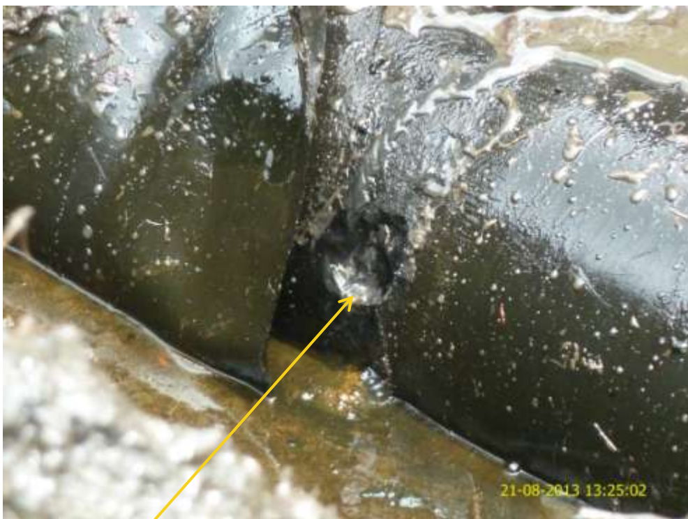
Close up: Drilled surface on 6" Cawthorne Channel Well45T flowline at Mbiama. Picture was taken during Joint Investigation of 21 st August 2013.
