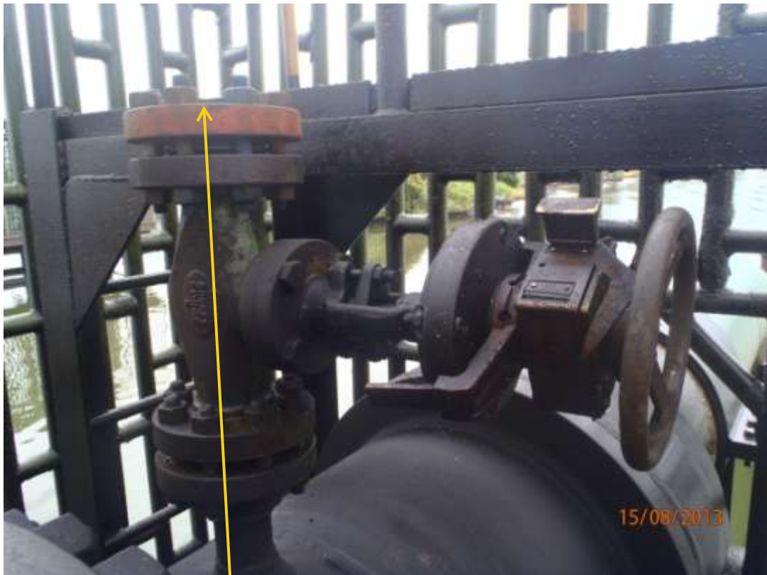
Close up: Position of missing pressure gauge at 24" Cawthorne-Channel loopline manifold at Ilomaturu. Picture was taken during Joint Investigation of 15 th August 2013.
