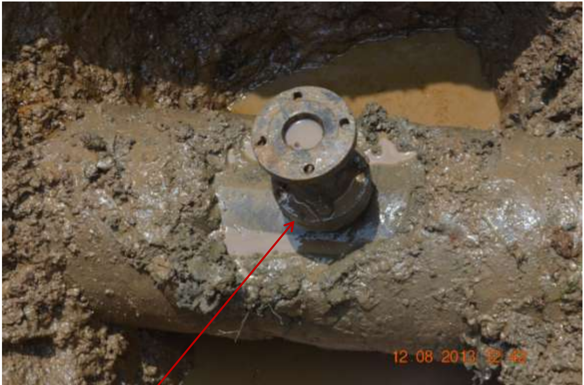
Close up: Illegal fitting on 14" Okordia-Rumuekpe pipeline at Akarimini. Picture was taken during Joint Investigation of 12 th August 2013.
