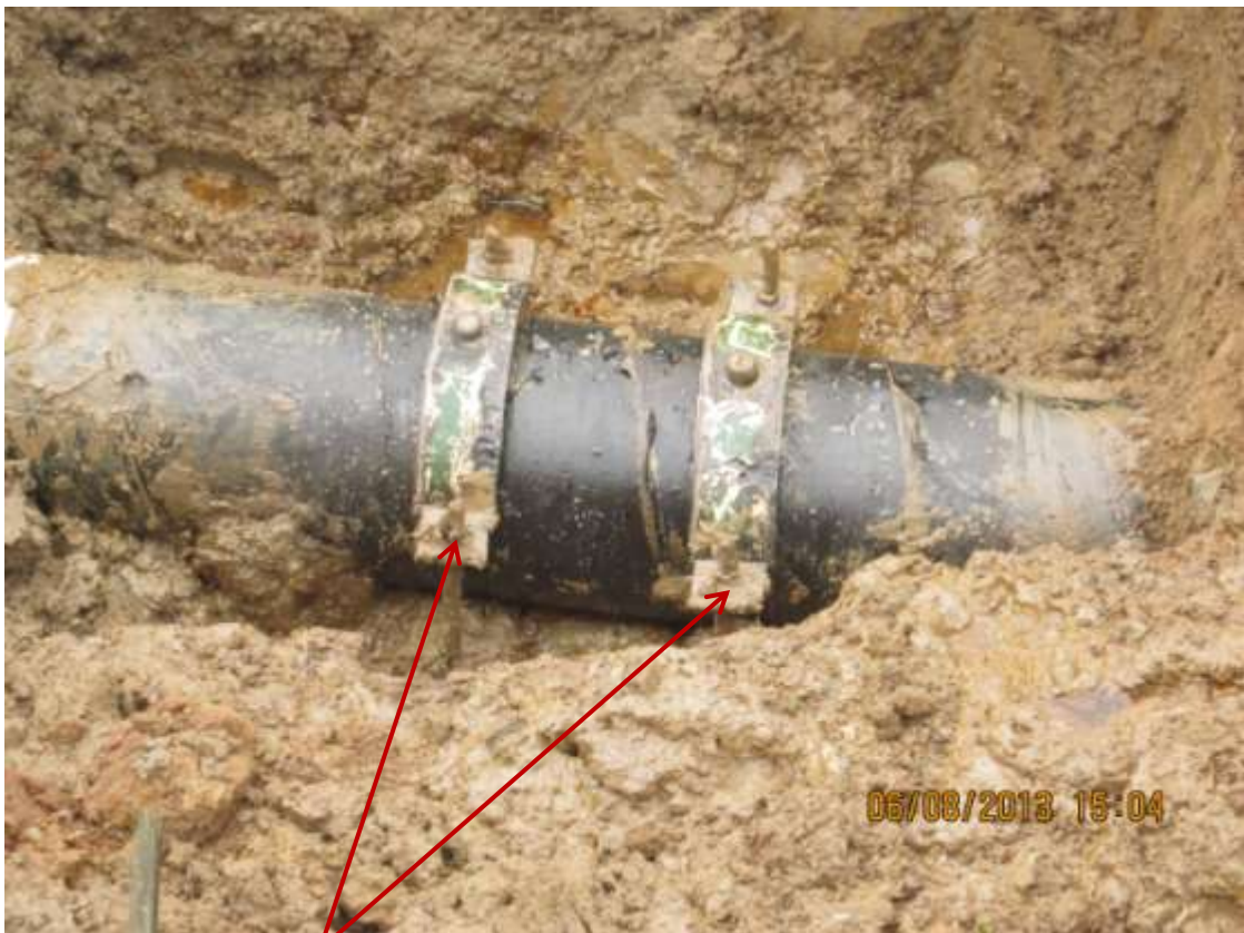
Close up: Illegal fittings on 12" Imo River2 – Ogale pipeline at Umuedeokwara/Odagwa. Picture was taken during Joint Investigation of 6 th August 2013.
