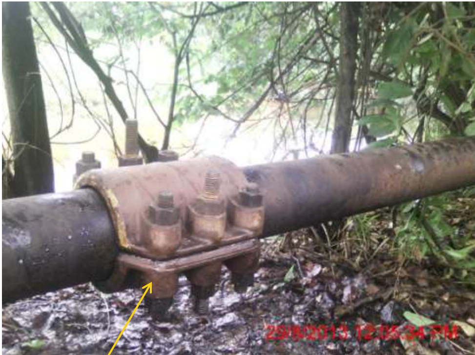
Close up: Tampered clamp on 4in Adibawa North East flowline at Biseni. Picture was taken during Joint Investigation of 29 th August 2013.
