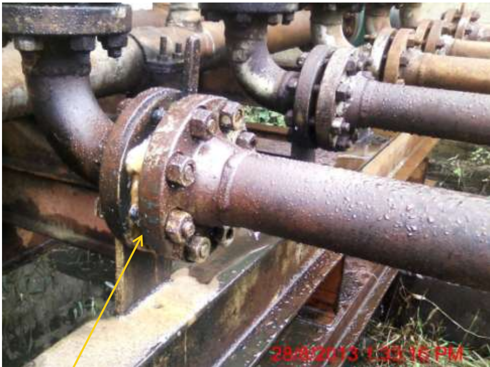
Close up: Leak due to gasket failure on Biseni Remote Manifold at Biseni. Picture was taken during Joint Investigation of 28 th August 2013.
