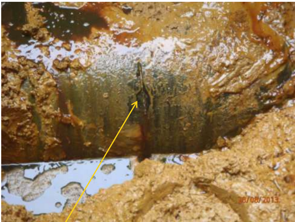
Close up Hacksaw cut on 16" Nun River – Kolocreek pipeline at Igiebiri. Picture was taken during Joint Investigation of 28 th August 2013.
