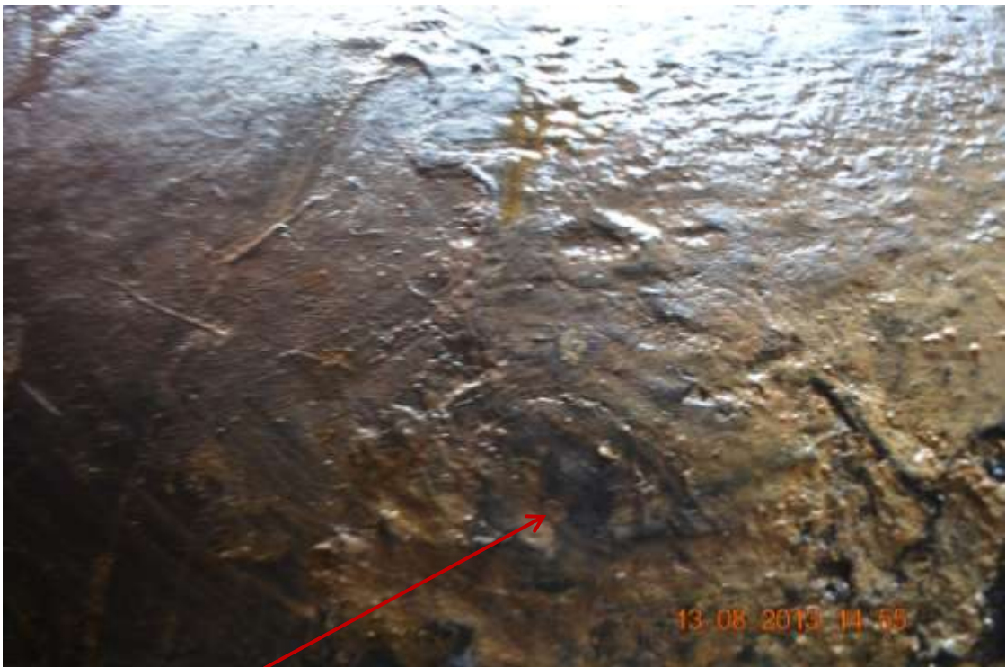
Close up: Leak due to corrosion at 6 o' clock position on 14" Okordia-Rumuekpe pipeline at Ikarama. Picture was taken during Joint Investigation of 13 th August 2013.
