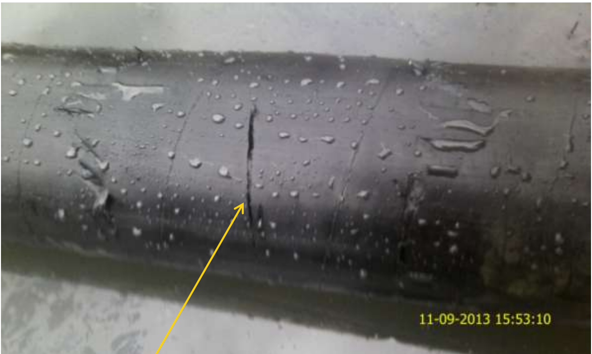
Close up: Hacksaw cut on Awoba Well3S flowline at Bille. Picture was taken during Joint Investigation of 11 th September 2013.
